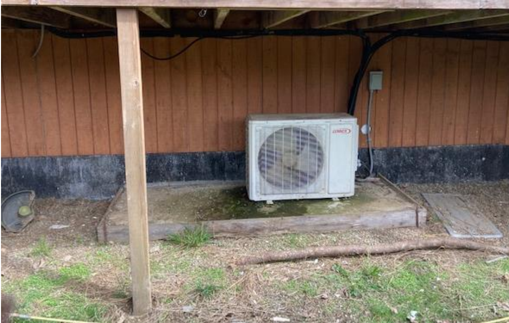
Photo 4: A heat pump, located at the rear of the primary residence, is the building's main source of heat.
