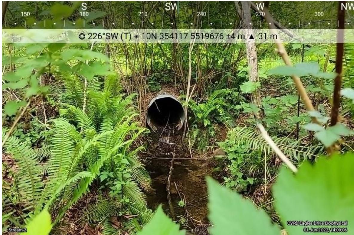
Photo 5. Hanging culvert that drains the road ditch. The channel is disconnected downstream and flows appear to entirely infiltrate into the ground.
