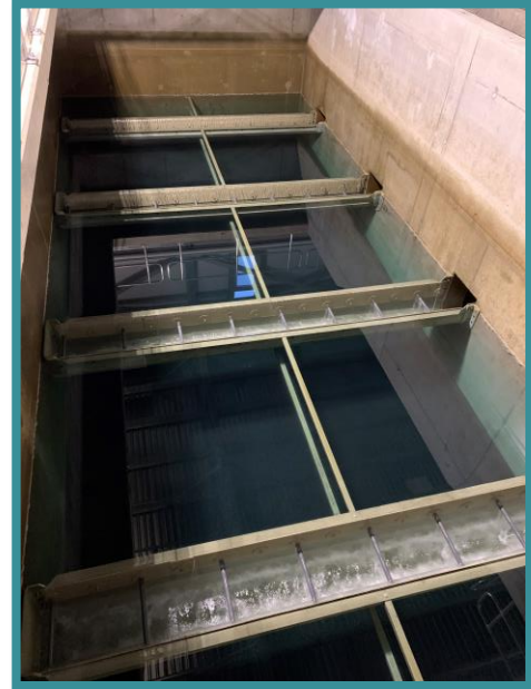
One of five filter beds at the treatment plant.
