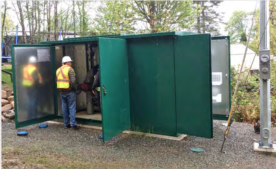
PRV Station - Nelson St at 4 th St
