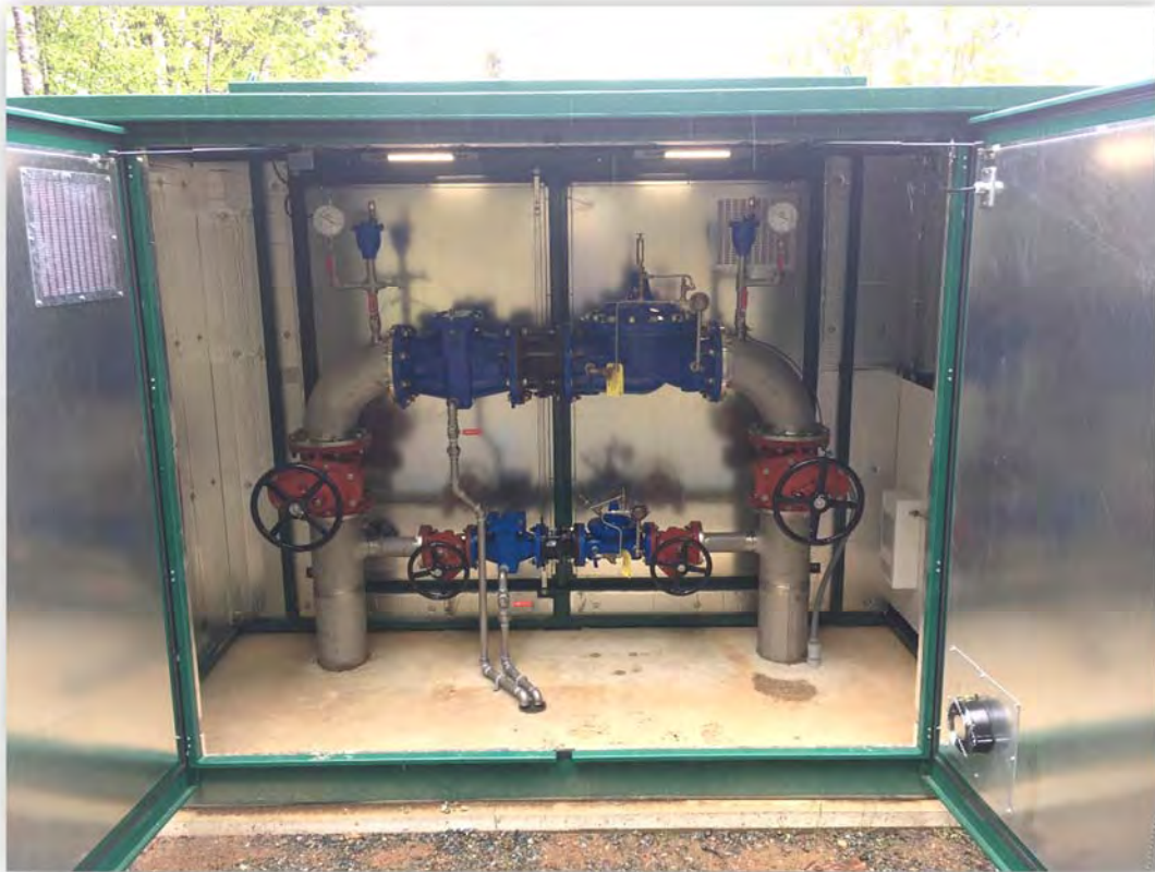
PRV Station - Nelson St at 4 th St (200 mm dia. & 75 mm dia.)
