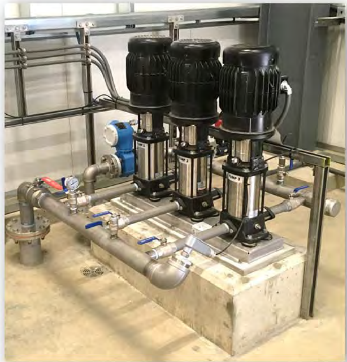
Booster Pump Station (PZ 155) Three Grundfos CR-5 Pumps
