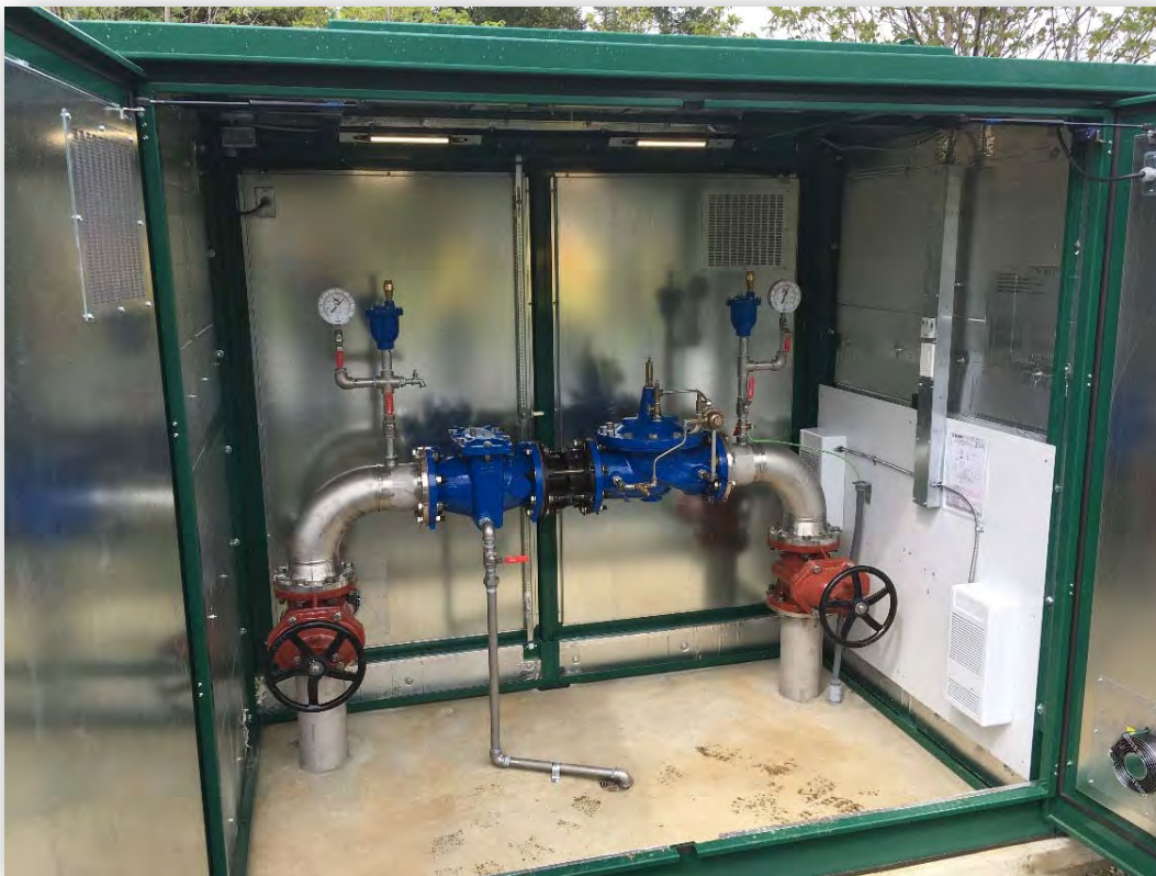
PRV Station – McLeod Rd at 4 th St (150 mm dia. & Low Flow)
