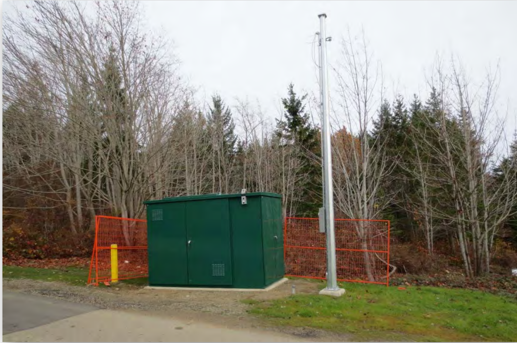
PRV Station – McLeod Rd at 4 th St
